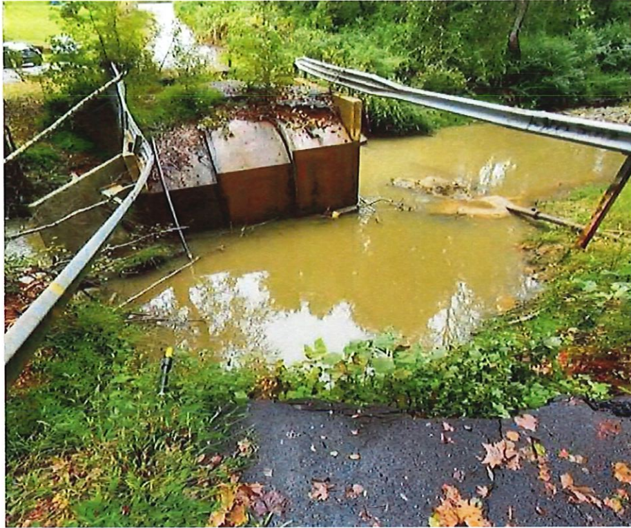
Photograph of the Snow Creek Bridge taken after Mr. Paxson's incident
